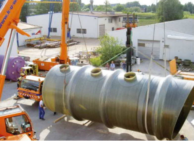
GRP Cooling water system DN3600 RWE Eemshaven
