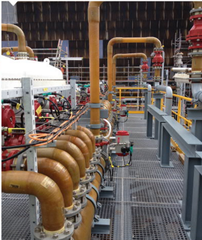
Piping chlorine system
